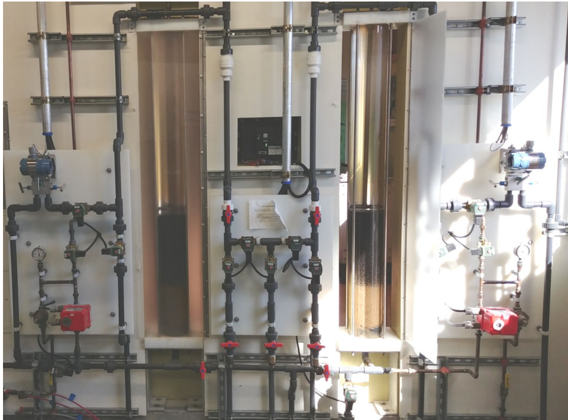
Control and Chlorinated Pilot Filters
