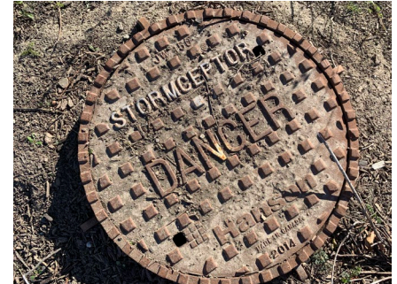
Oil Grit Separators
