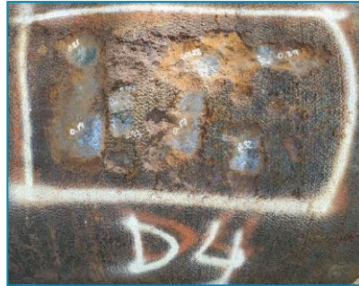
Validated Pipe Defect
