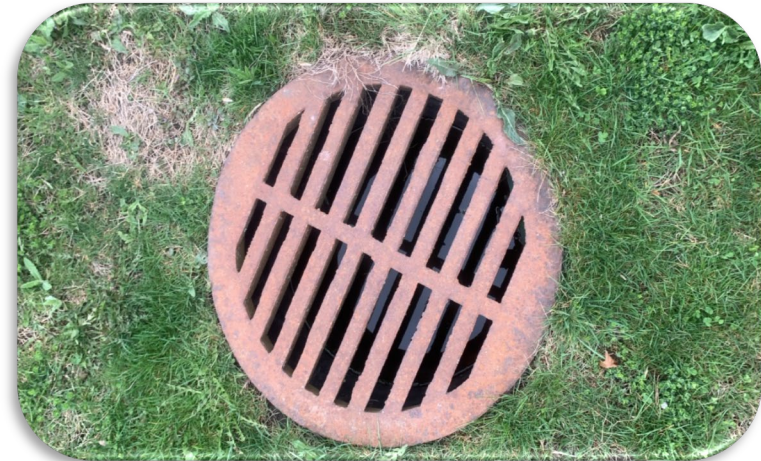
Example of a catch basin identified in North Woodslee – 2023
