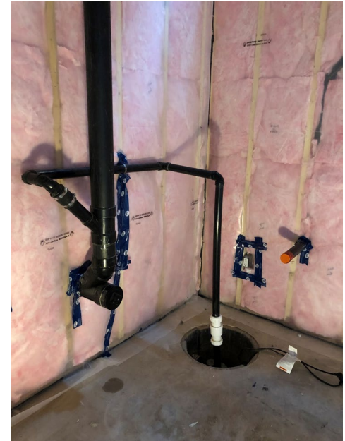
Sump water illegally connected to the sanitary sewer
