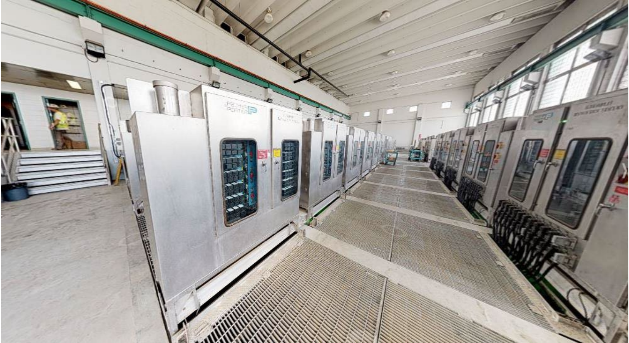
Old UV Disinfection System
